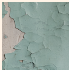
Peeling lead paint
